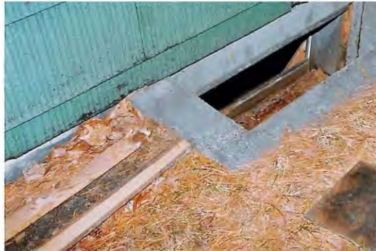
Photograph 3 of the boards used to secure the window from the inside 11
