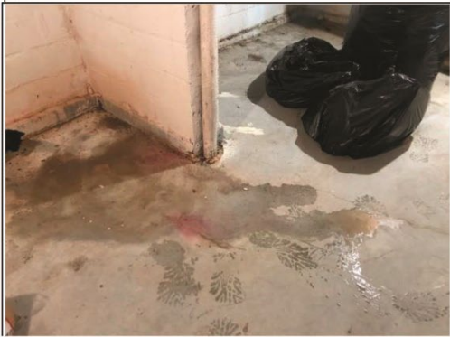
HIS757: Water in basement, repair not made
